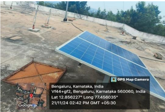
Solar Panels at Mechanical Department
