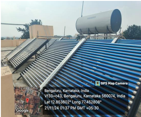
Solar Water Heaters at VKIT Girls Hostel
