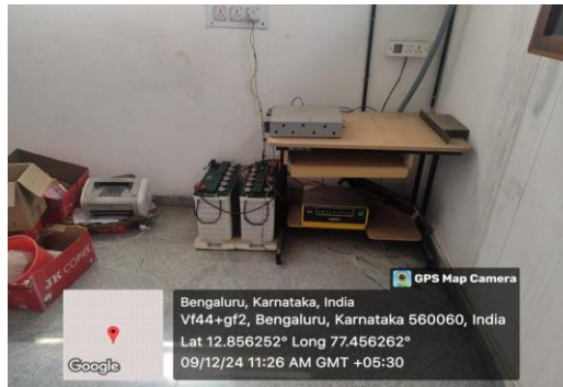
Battery Storage of Power Generated From Solar Panel
