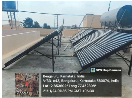
Solar Water Heaters at VKIT Boys Hostel
