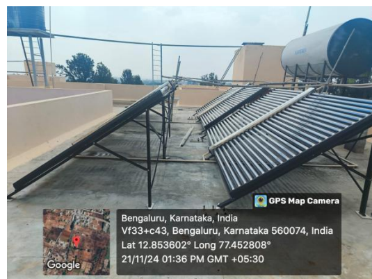
Solar Water Heaters at VKIT Boys Hostel
