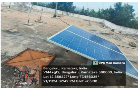
Solar Panels at Mechanical Department
