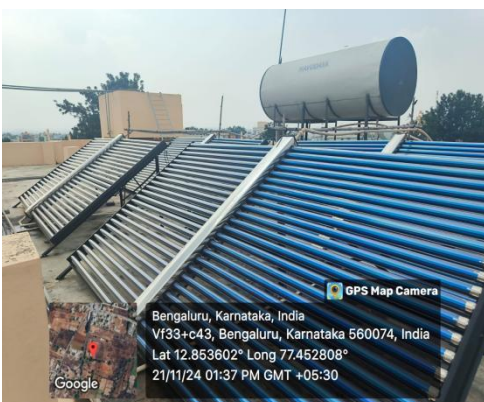
Solar Water Heaters at VKIT Girls Hostel
