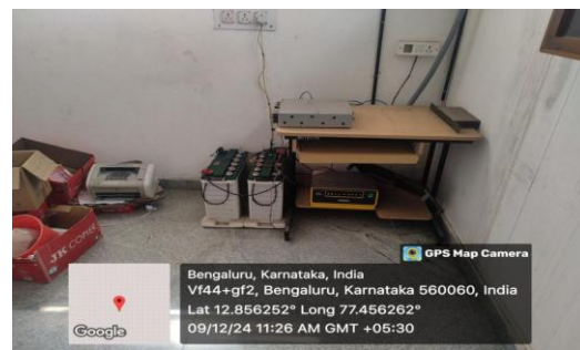
Battery Storage of Power Generated from Solar Panel
